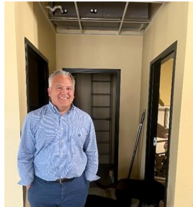
Ted Kanelopoulos in the new McGree Admin wing at La Salle HS in Yakima
